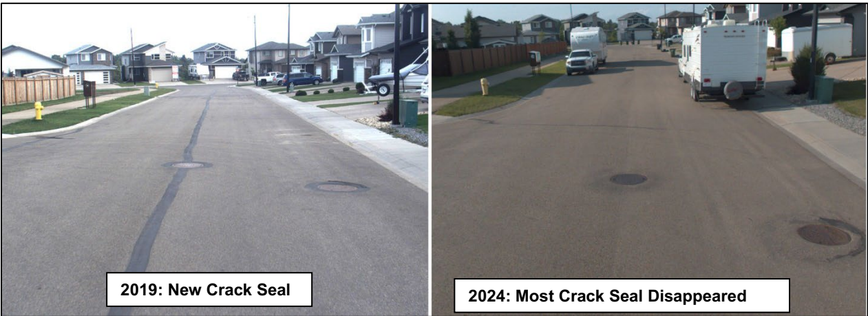
Figure 8: Example of Local Roads Showing PCI Improvement as Crack Seal Fades
