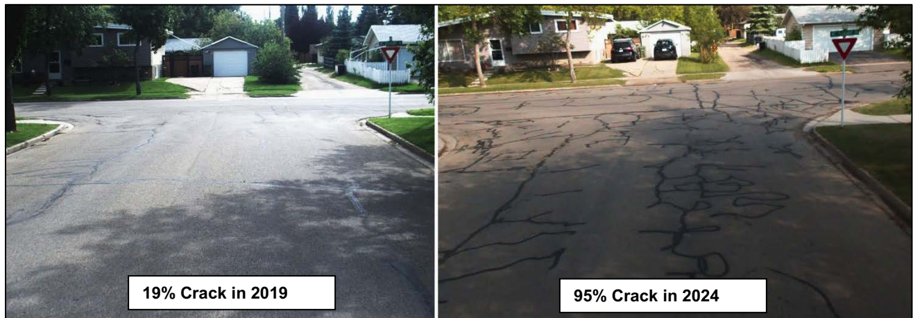
Figure 6: Example of Roads with Increased Crack Sealing in 2024 Compared to 2019
