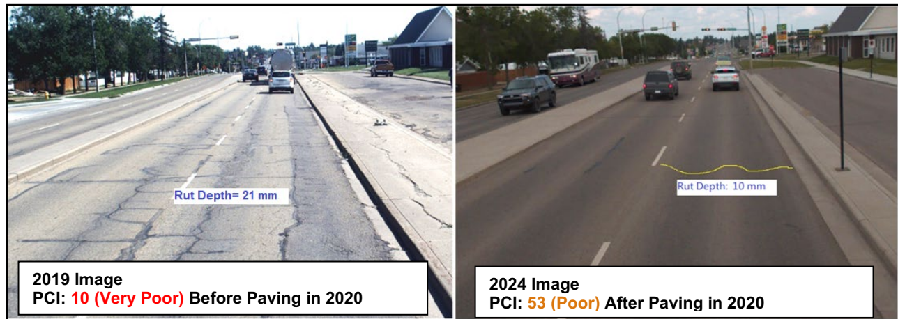
Figure 7: Example of Arterial Road (48 Avenue) with Rut Issue Before and After paving
